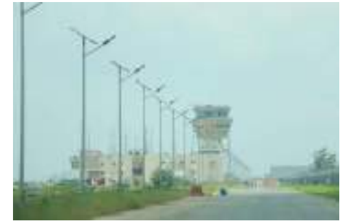
Over 800 Solar Lights - Airside
