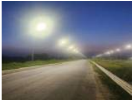
Smart on-demand illumination leading to Energy Conservation
