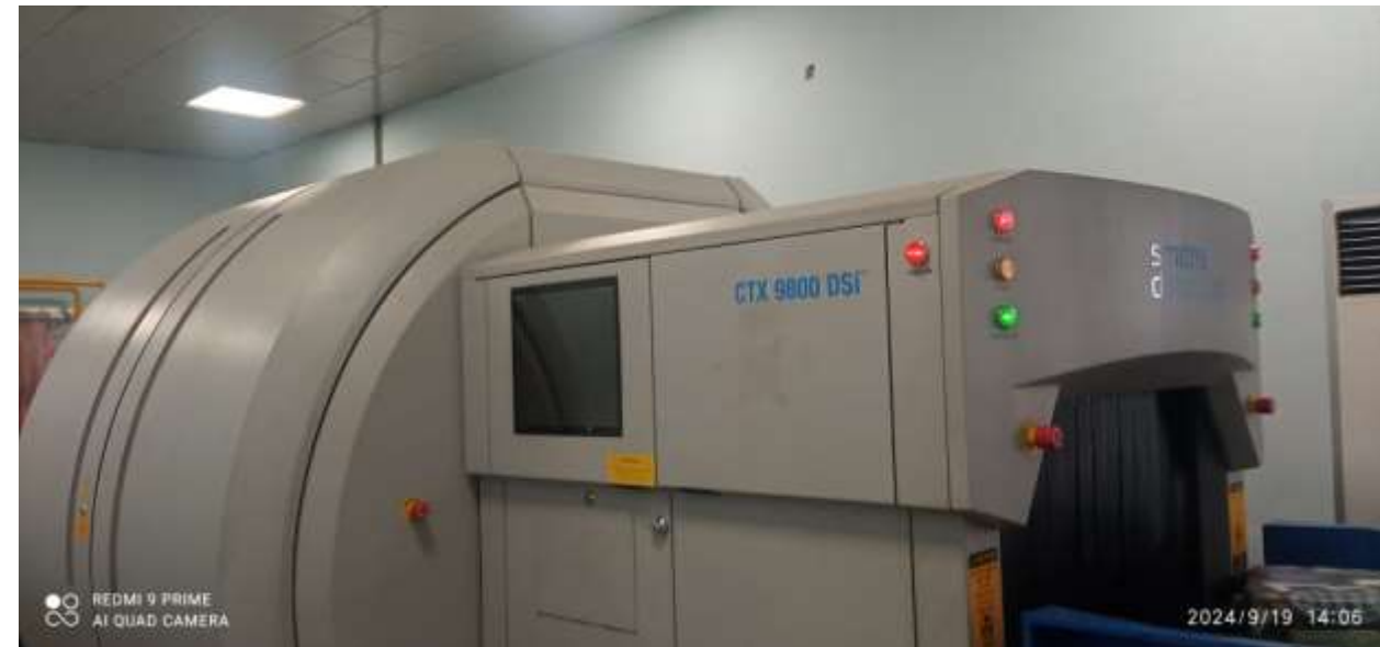
D.1 Inline Baggage Screening System (ILBS)
